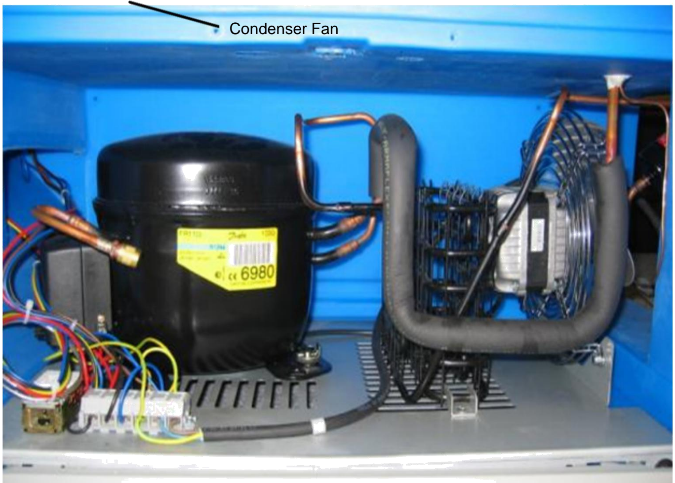
Figure 36. Condenser and its surrounding, physical photo
