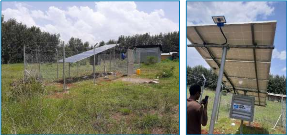
Figure 18: Solar Powered Water Supply system
