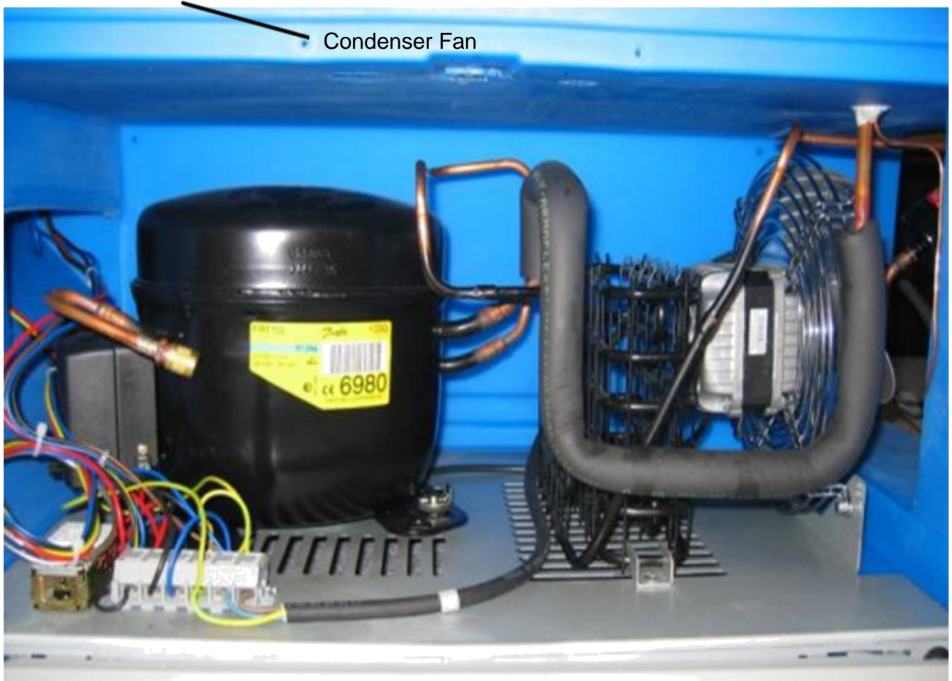
Figure 36. Condenser and its surrounding, physical photo
